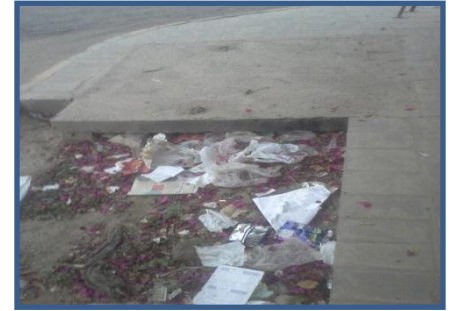
Plastic bags clogging drains, Al-Asbahi
